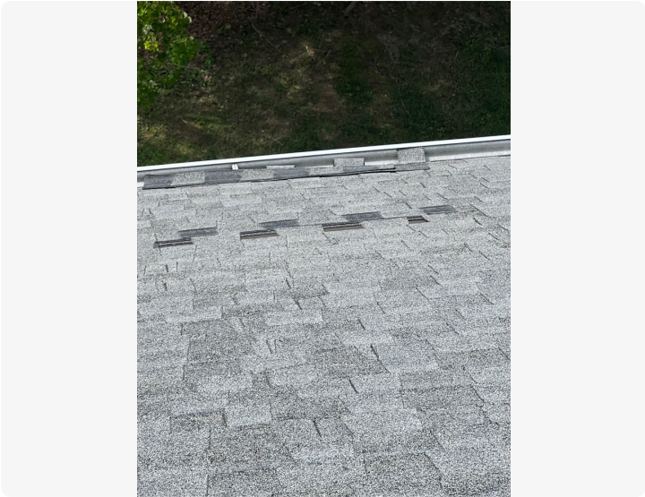
Multiple sections of missing shingles are visible on the rear slope of the roof.
