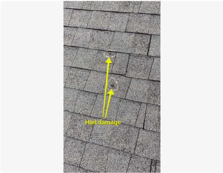
Existing hail damage chalked. Limited hail damage found throughout roof but a new notable hits. These circled ones are down to the fiberglass mat and will shorten the lifespan of the shingles.
